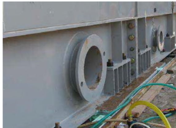
Figure 1. Saturating and draining the excessive water in the anchor holes of the turbine foundation prior to grouting.
